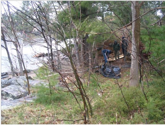
Plate 13: View to northwest showing drilling rig on “dressed and levelled site” of 1924 Bala No. 2 power station.
