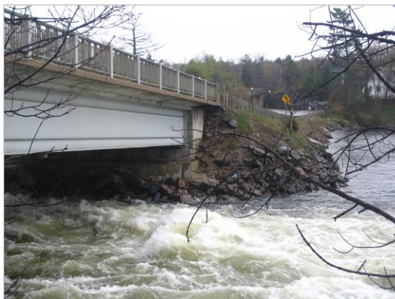
Plate 15: View across channel of South Bala Falls with rock filled road bed covering a granite point extending out from the shore.
