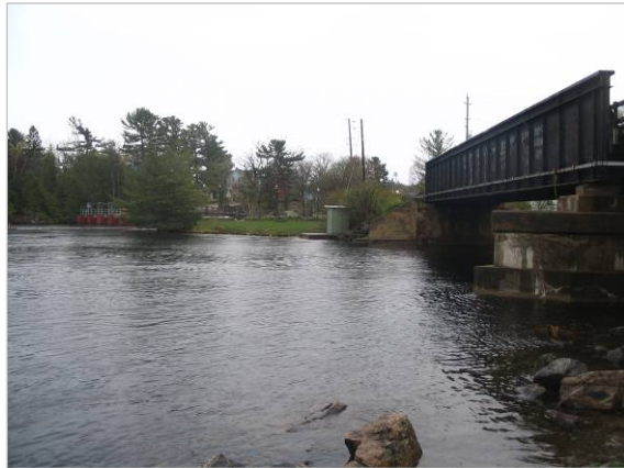
Plate 3: 1908 CPR bridge over North Bala Falls channel. Note small parkette just east of rail embankment.
