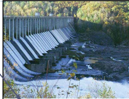
Remotely-operated dam gates can quickly turn calm waters or dry riverbeds into dangerous flows.
