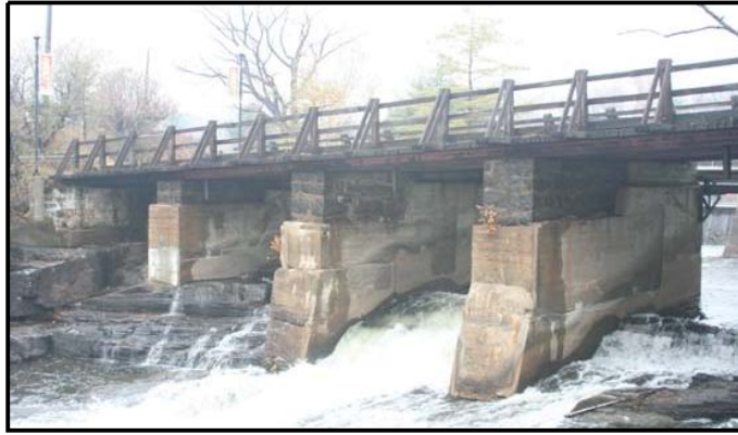
Figure 34 Six span Bala Road Bridge over South Channel with remnant of 1913 dam.
