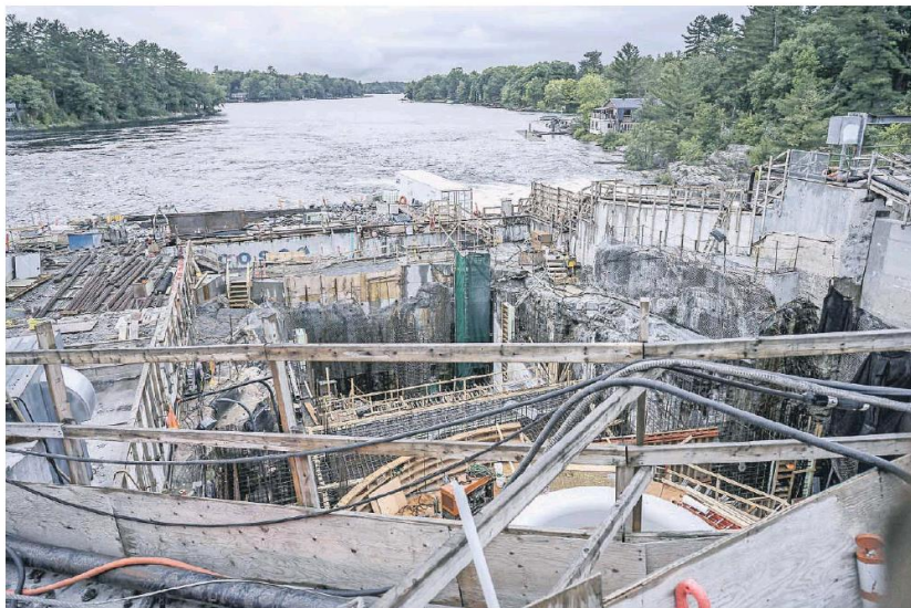
Work continues on the North Bala Small Hydro Project in Bala, Ont., on Wednesday, despite Premier Doug Ford's campaign promise to cancel the project, which he has now reversed. Mr. Ford now says terminating construction of the power station would be too expensive. J.P. MOCZULSKI/THE GLOBE AND MAIL
