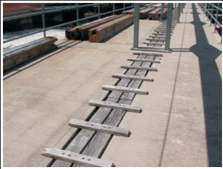
DAM DECK WITH UNSECURED STOPLOG GAIN COVERS
